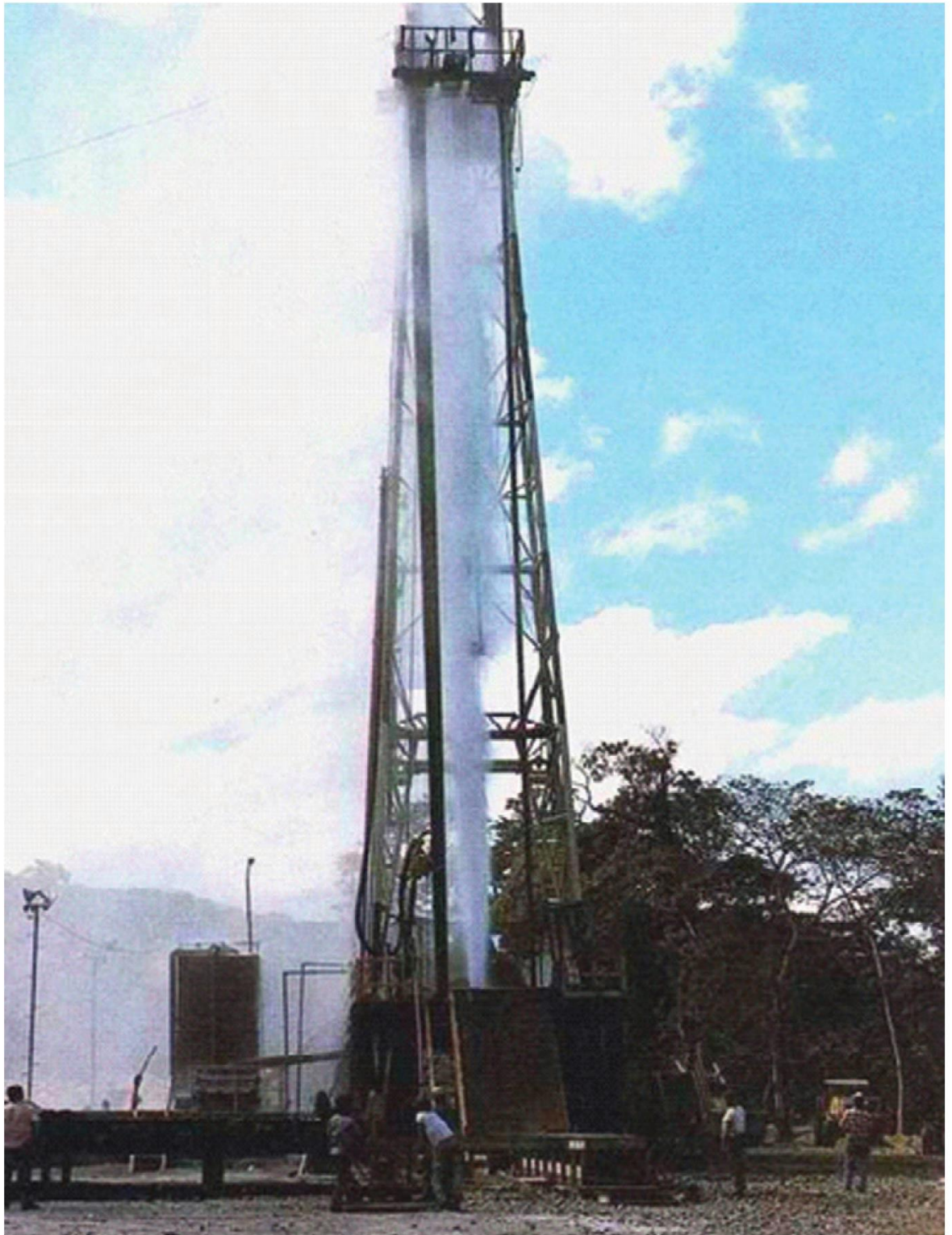
Fig. 3.1 Discharge from a well at the Ahuachapán field, El Salvador [1] [WWW].
