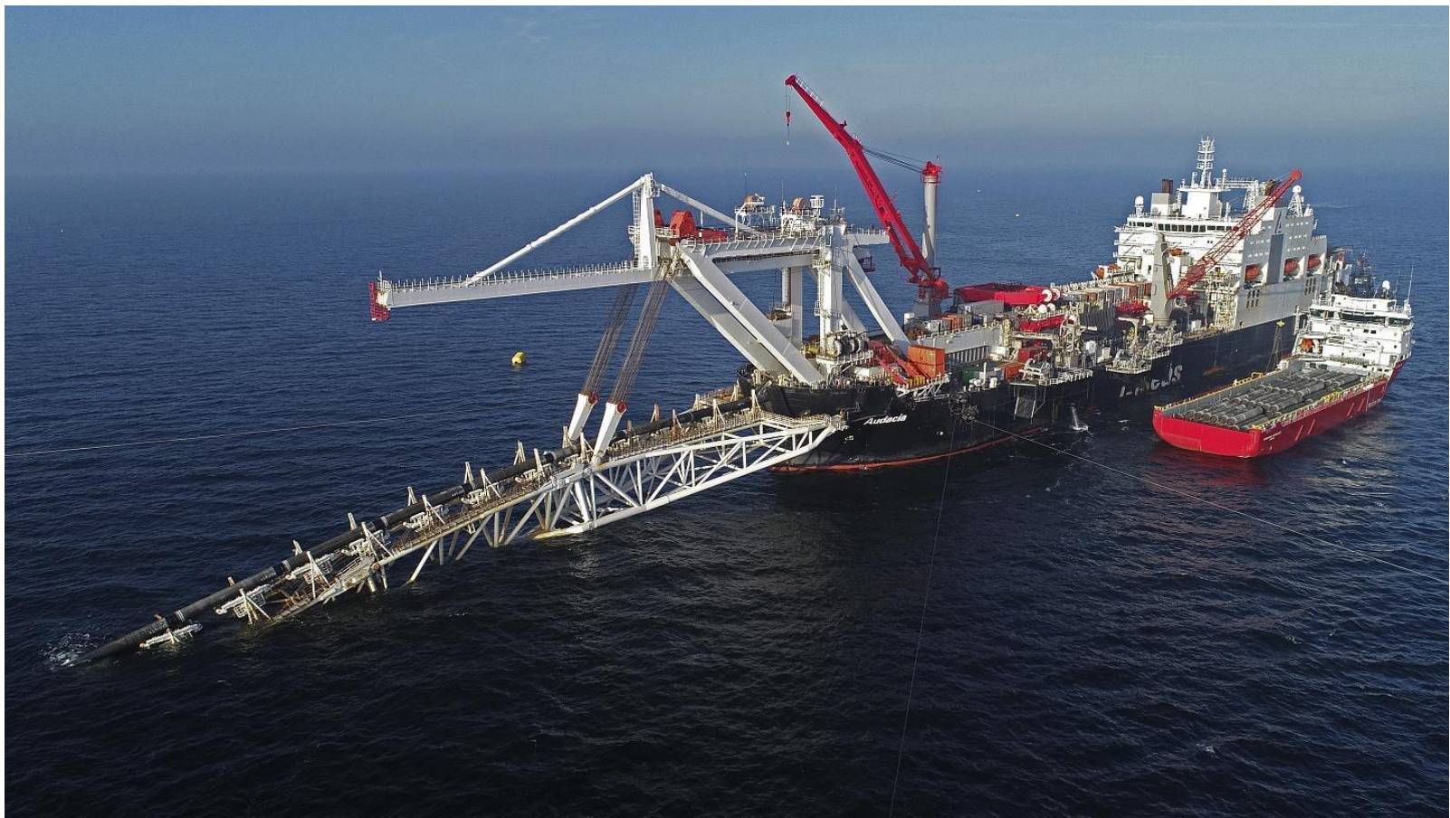
A specialized barge lays pipe under the Baltic Sea in 2019 for the controversial Nord Stream 2 pipeline, which is meant to carry additional Russian gas to Germany
