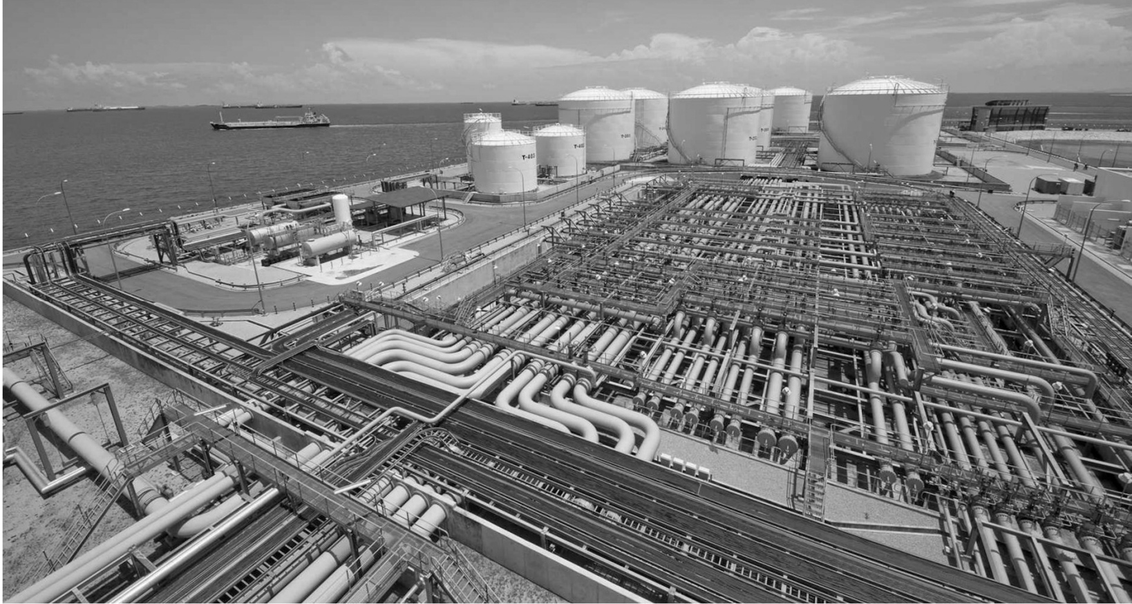
The oil terminal in the Port of Singapore.
