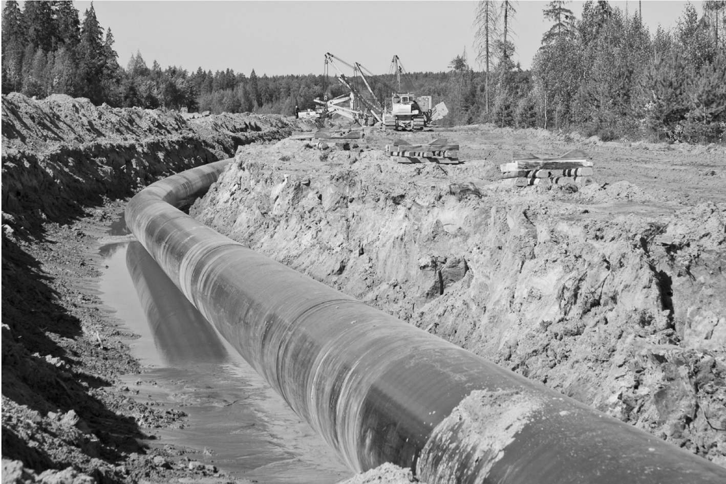
Pipelines are used to transport liquid bulk over long distances. Source: Vladimir Kolobov
